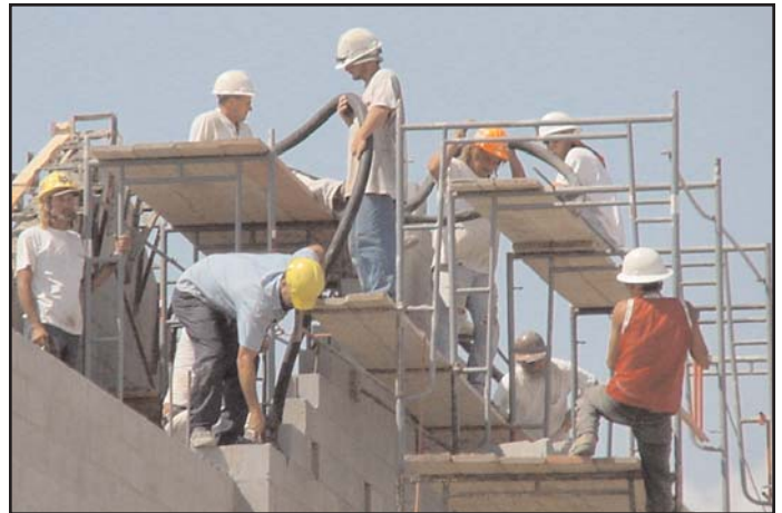
Above scaffold shows violations typically found at construction sites: workers are not wearing safety harnesses, platforms are not fully planked, and there is no guardrail system.
