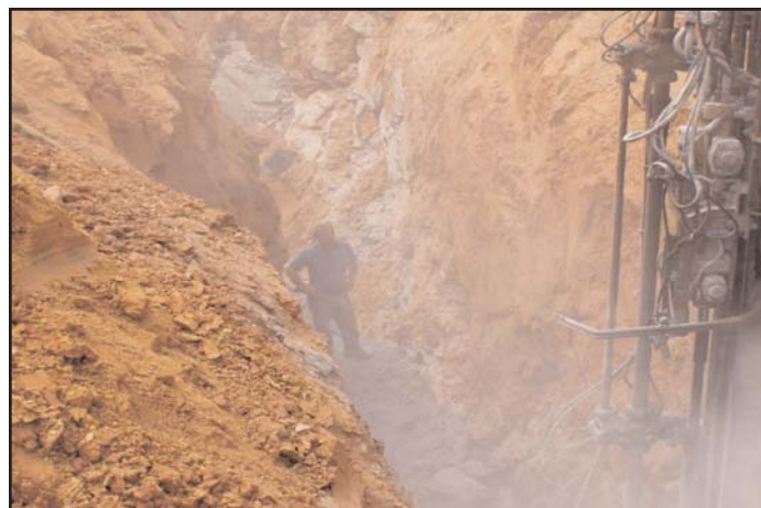
An employee works in a 20-foot-deep unprotected trench while observing the drilling of a hole before he packs it with dynamite for blasting. The employer should provide a trench box or shoring to protect the employee from cave-in.
