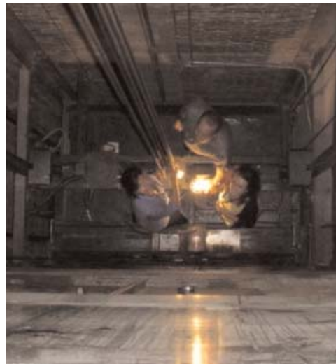
Elevator inspectors open the elevator shaft during routine inspections. Over 20,000 elevators and escalators are inspected each year by NCDOL.
